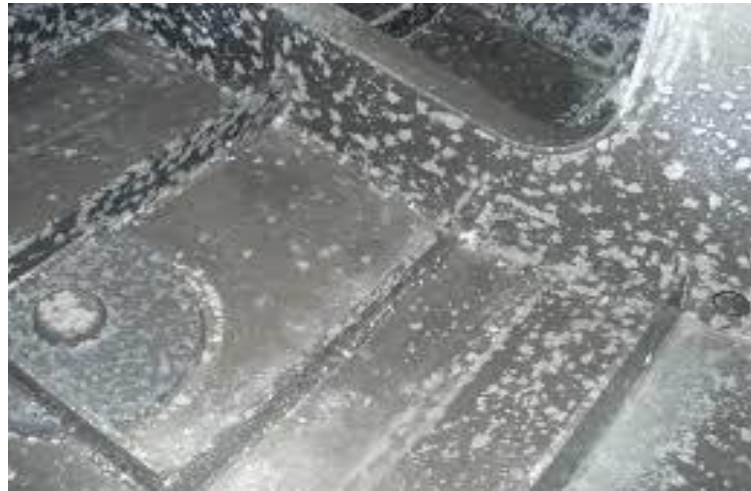
Fig 4: Pitting in aluminum
