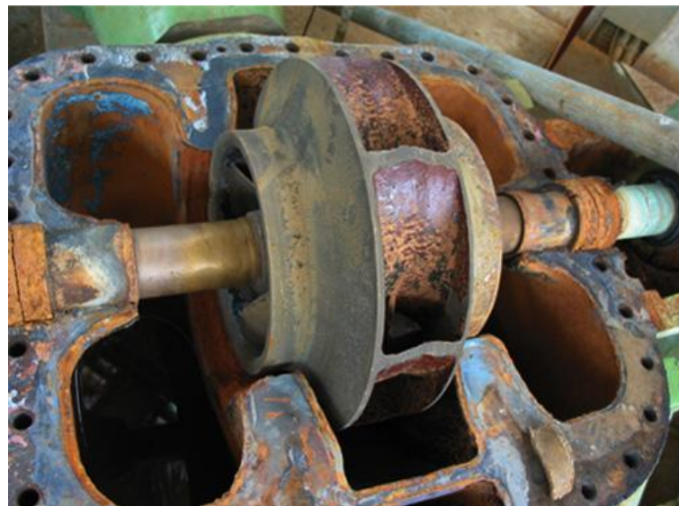
Figure 2: Erosion Wear of Impellers.
