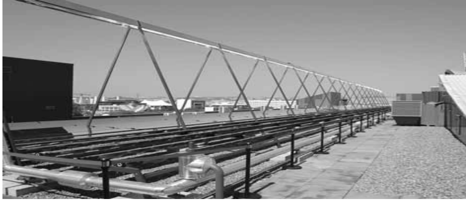
Figure 2.26. The third Industrial Solar project operating temperature 180°C [61].
