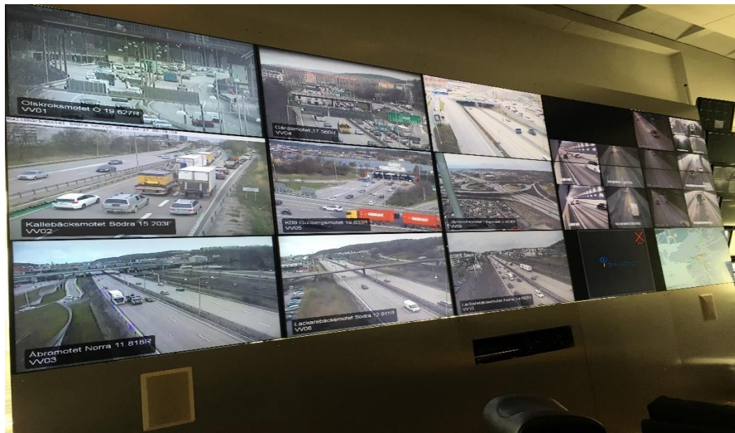
FIGURE: 3.17 Traffic Management Centre (TMC)
