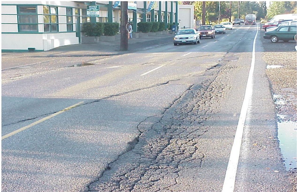
Figure 2.2 Severe mix rutting
