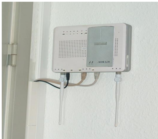
Fig.-4.11 Wi-fi router attached on the wall
