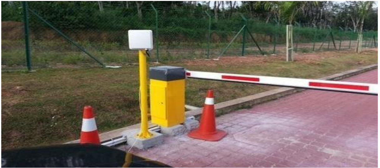
Fig-4.16 RFID reader and Boom Barrier
