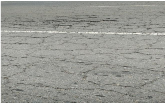
Fig.32: Block Cracking near Phagwara bus
