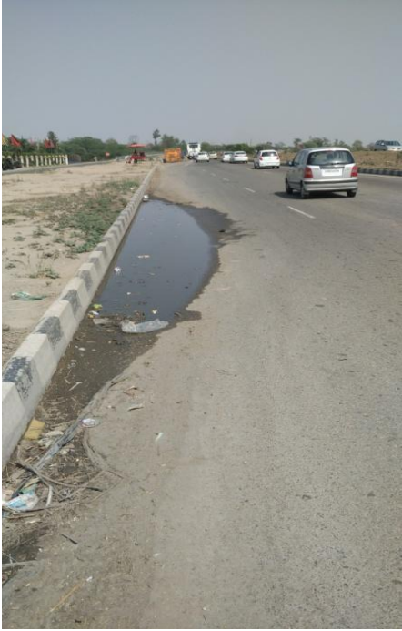
Fig. 3: Water on the existing road.
