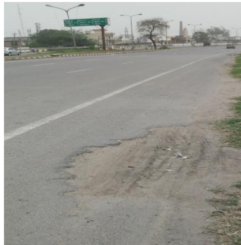
Fig.17: Edge cracking at Phagwara (near sugar mill)
