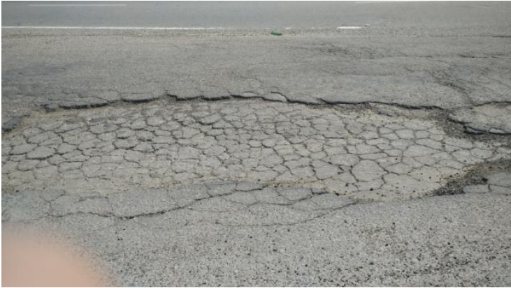
Fig.4: pothole with cracks on road near Chaheru.
