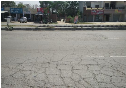
Fig.33: Alligator cracking near Virk Village
