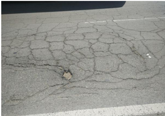
Fig.31: Slippage Cracking Civil Hospital stand
