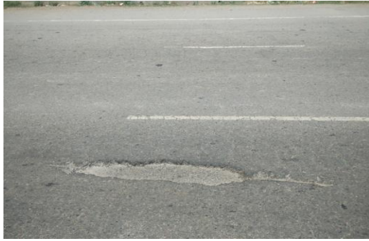
Fig.29: Potholes near Chak Hakim
