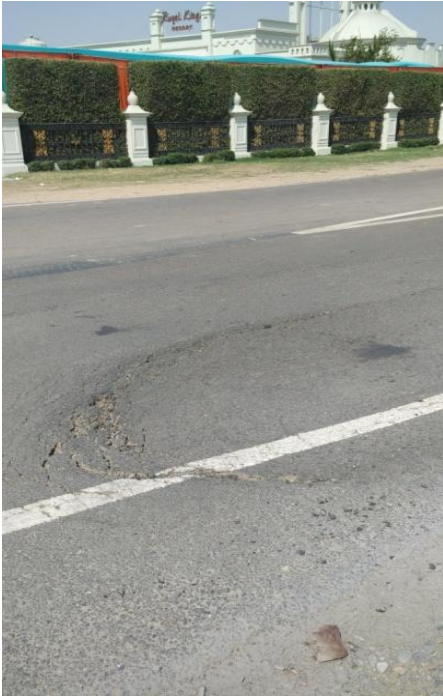
Fig. 2: Slippage cracks near Royal Pesort.
