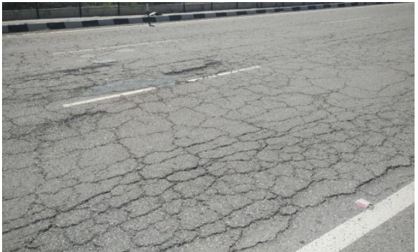
Fig.34: Alligator Crracking near Mouli Village.
