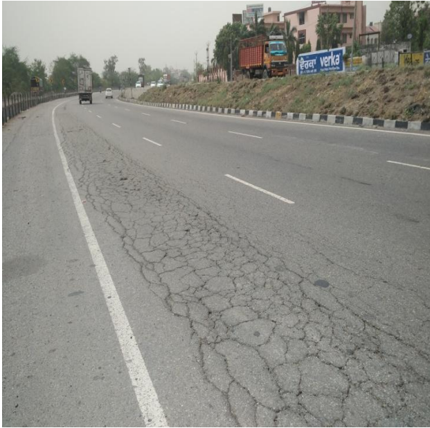
Fig.21: Alligator Cracking near DAV College
