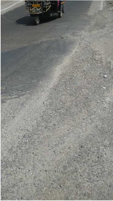
Fig.14: Patches and revealing near LPU.
