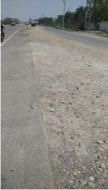
Fig.5: No drainage system.
