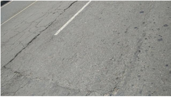
Fig.30: Block Cracking near Chak Hakim
