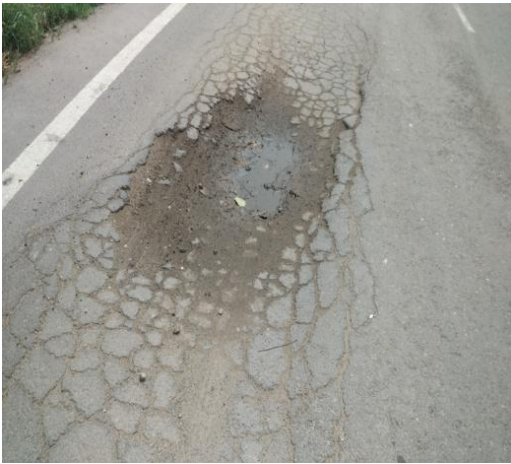
Fig.16: Rutting and cracks at Kajurla (near Havelli).
