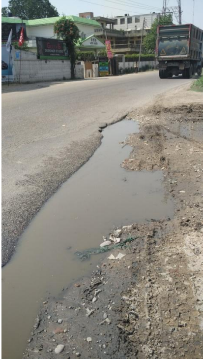
Fig.11: appearing edge cracking
