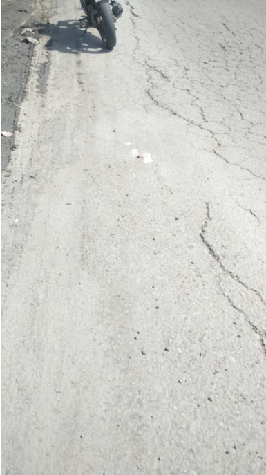
Fig.10: Pumping and cracks near Mouli
