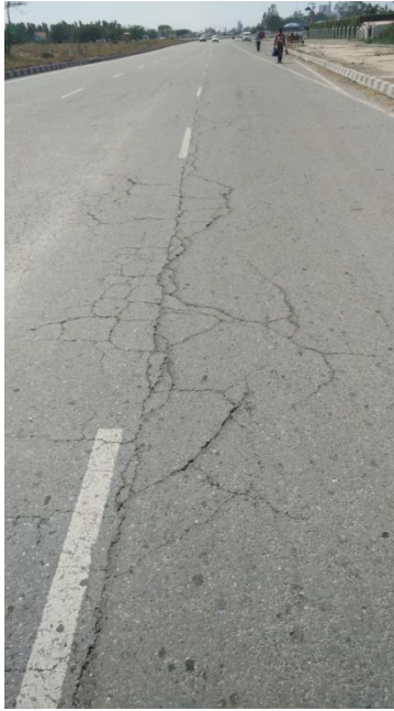
Fig.15: longitudinal cracking at chaheru.
