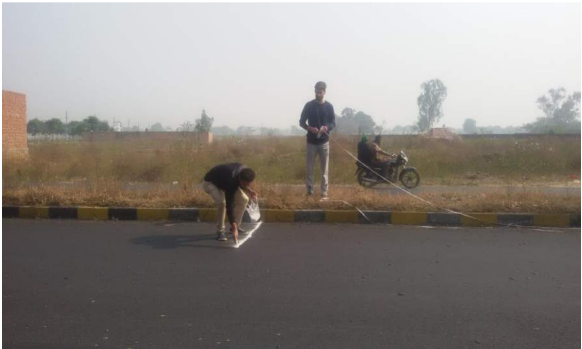
Fig.3.41: marking reference lines on the stretch (Rama Mandi-Hoshiarpur) NH-3(source: image taken by camera phone)
