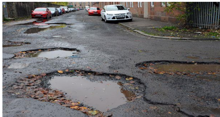
1.4:- Potholes on roads
