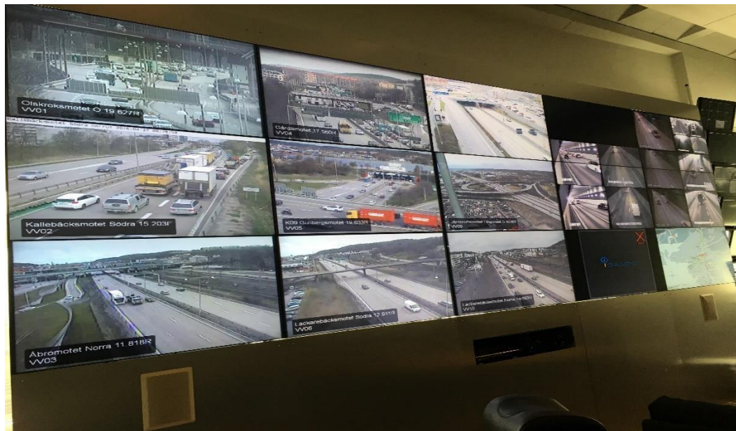
FIGURE: 3.17 Traffic Management Centre (TMC)
