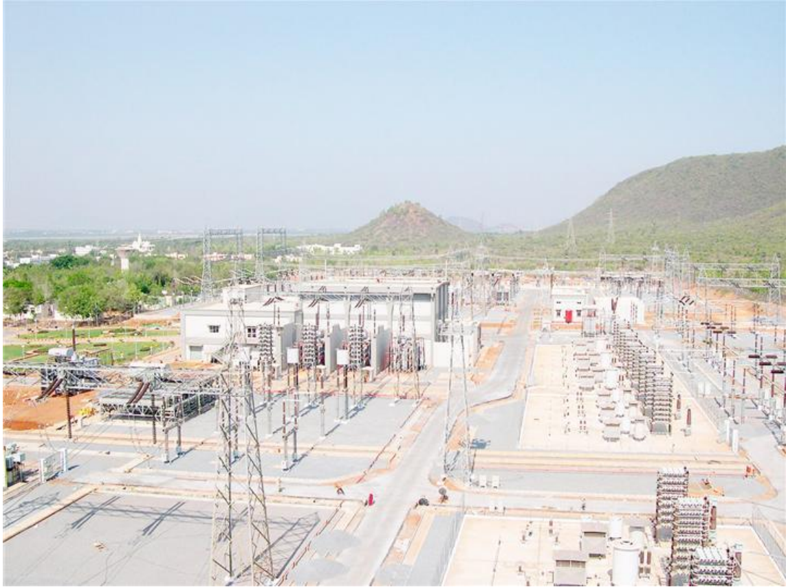
Figure 1.6- Vizag I and Vizag II HVDC Link.
