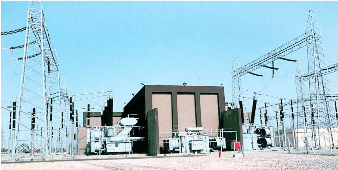
Figure 1.3- Vindhyachal HVDC Link.
