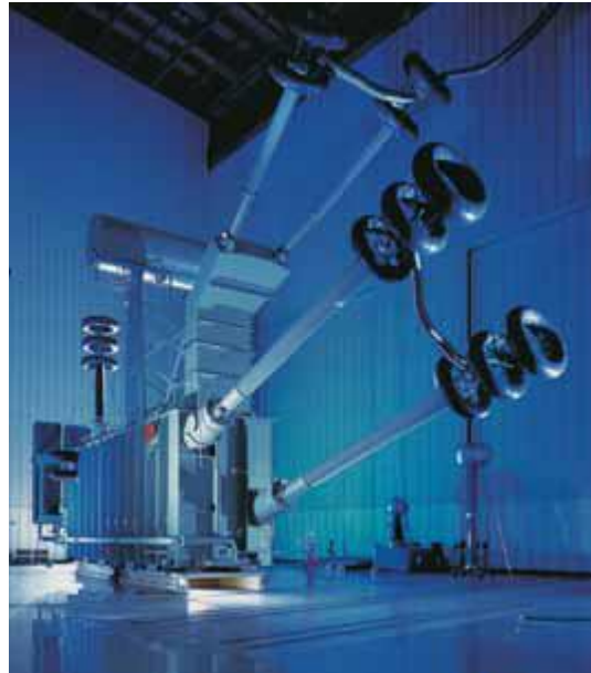
Figure 4.4- Converter Transformer during type test [34].
