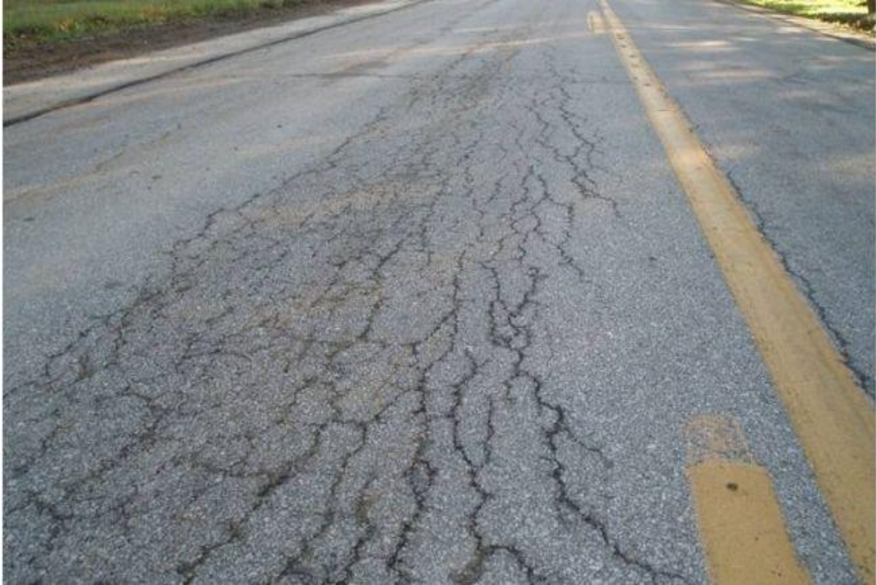
Figure 2.1 : Stripping on flexible pavement upper surface
