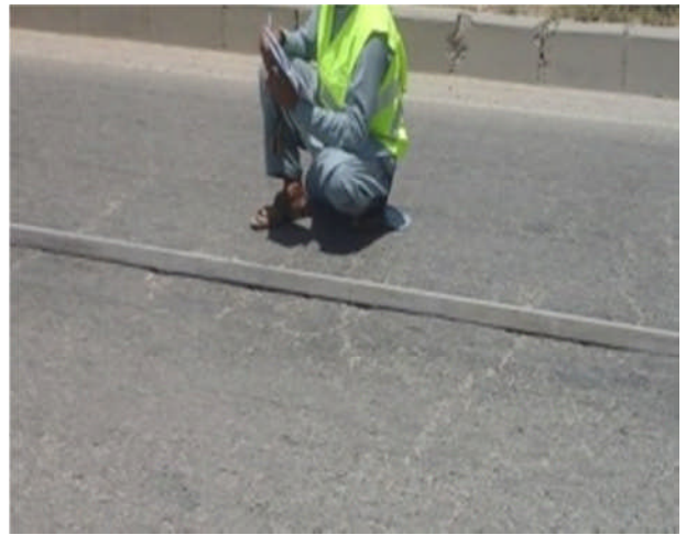
Figure8: Low Severity Corrugation
