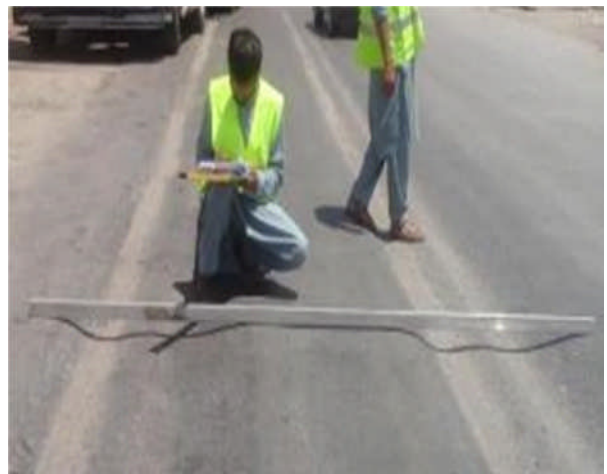
Figure16: High Severity Rutting
