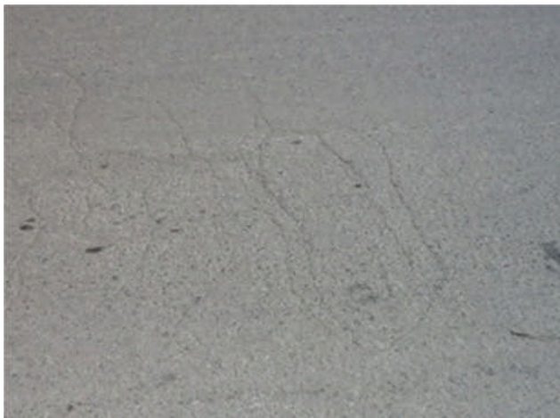
Figure13: Medium Severity Slippage cracking
