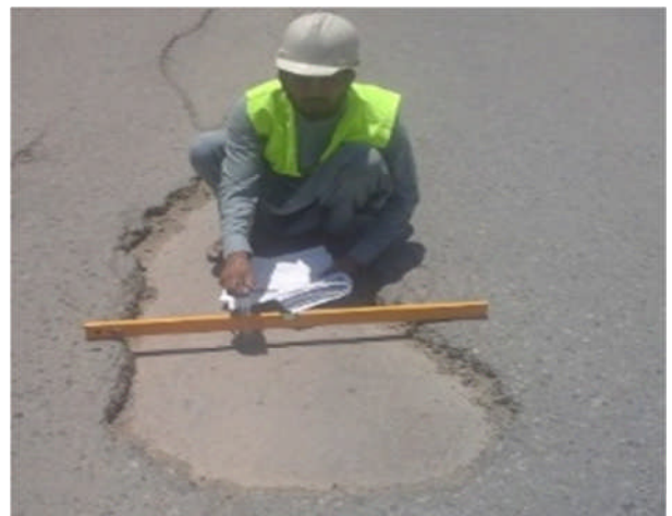
Figure10: High Severity Potholes
