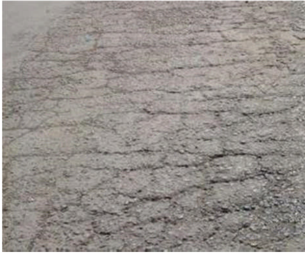
Figure5: Medium Alligator cracking
