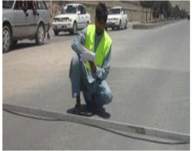
Figure12: High Severity Rutting
