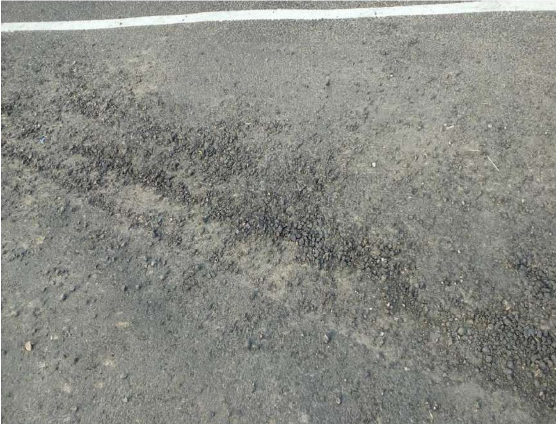
Figure 4-3: Loss of Aggregates
