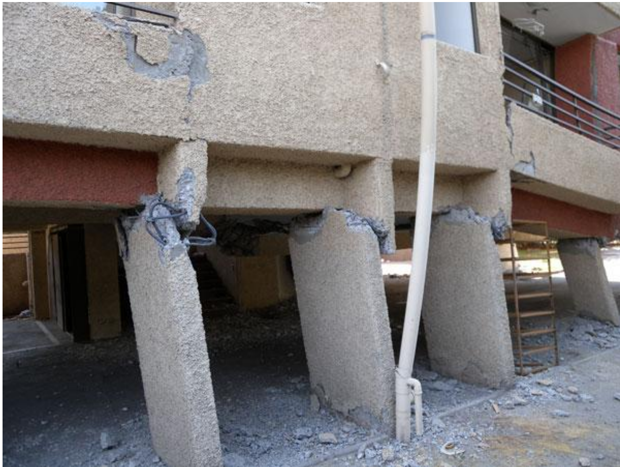
Fig 1 : Damage to columns at ground floor
