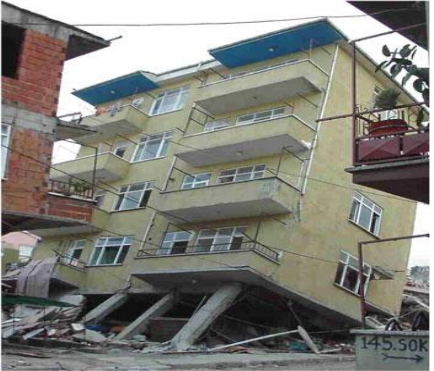
Fig 2 : Damage to columns in the soft storey
