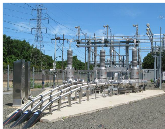
Installed HTS system
