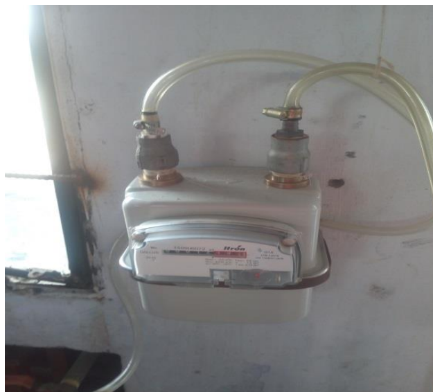
Figure 4.18 Manual biogas mass flow meter
