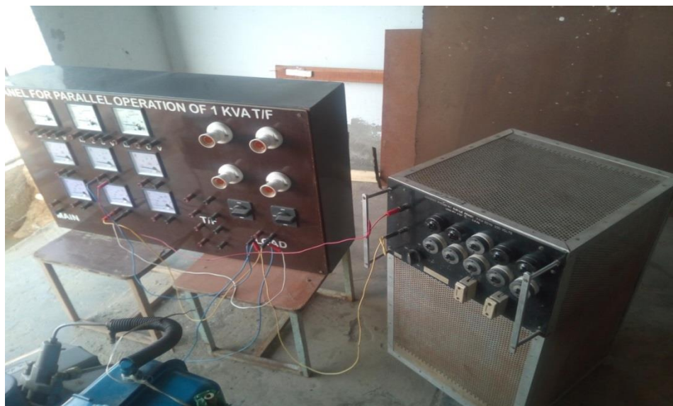
Figure 4.16 Load bank with electrical panels
