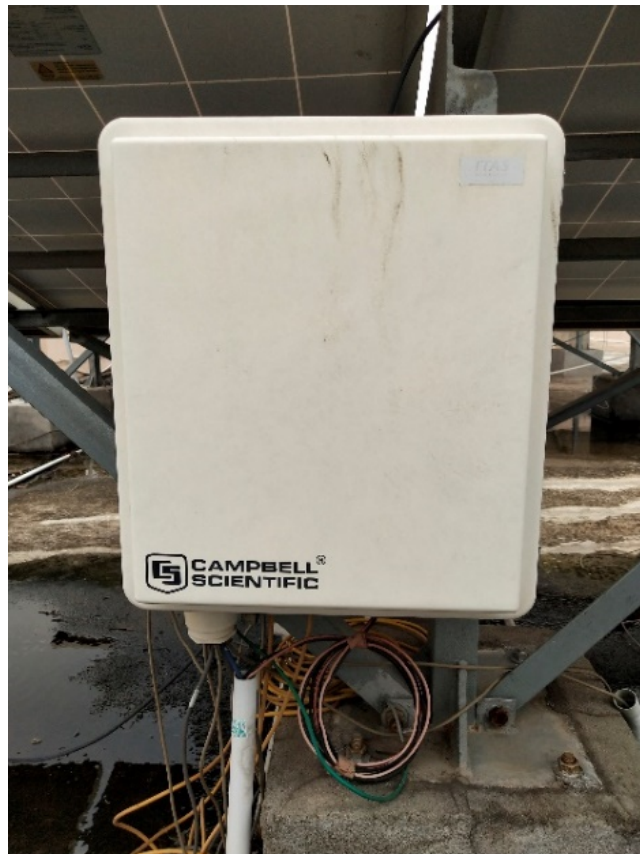
Fig. 2.3 CR3000 Data Logger
