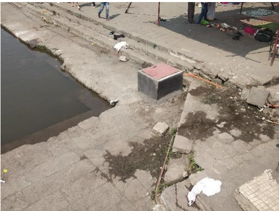
Image 4.53 Broken steps not repaired
