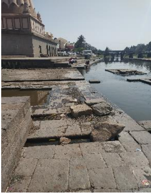
Image 4.11 Broken elements on the Dharmapuri ghats, Wai
