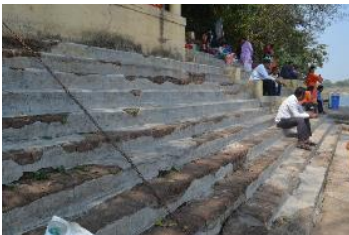
Image 4.37 Brick construction: Lower steps worn out due to floods every year
