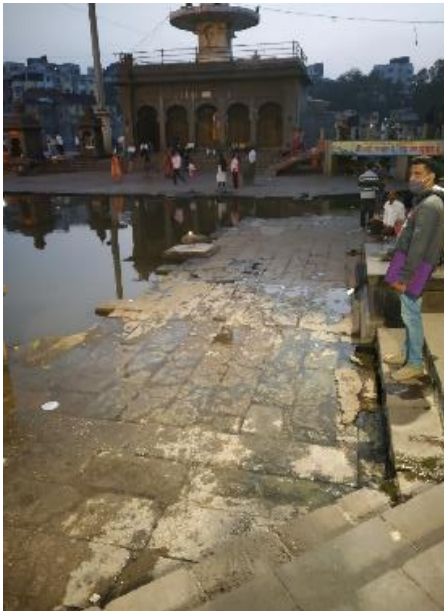
Image 4.47 Dangerous steps at the lower level of ghats.
