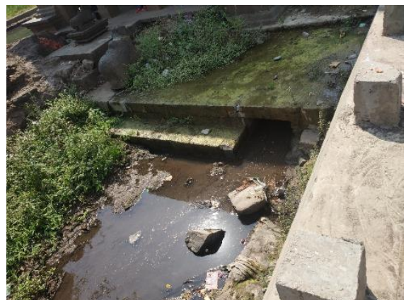
Image 4.14 Stones have fallen apart and laying around on Ganpati ghats, Wai.
