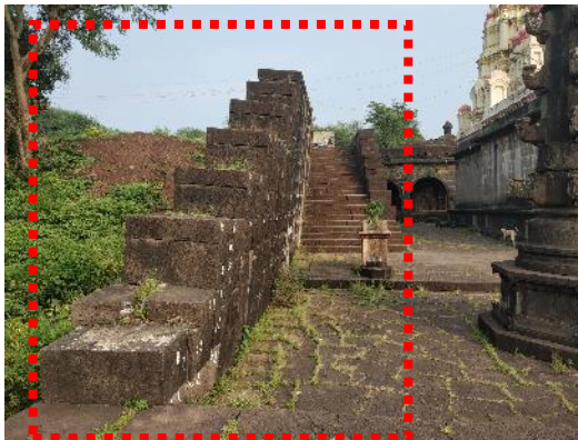
Image 4.21 Damaged steps at Sangam Mahuli
