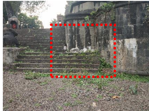
Image 4.20 broken steps at Sangam Mahuli ghat
