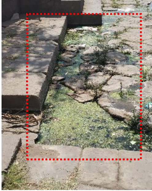
Image 4.7 Open sewer led in between the steps of the ghats at Gangapuri ghats, Wai
