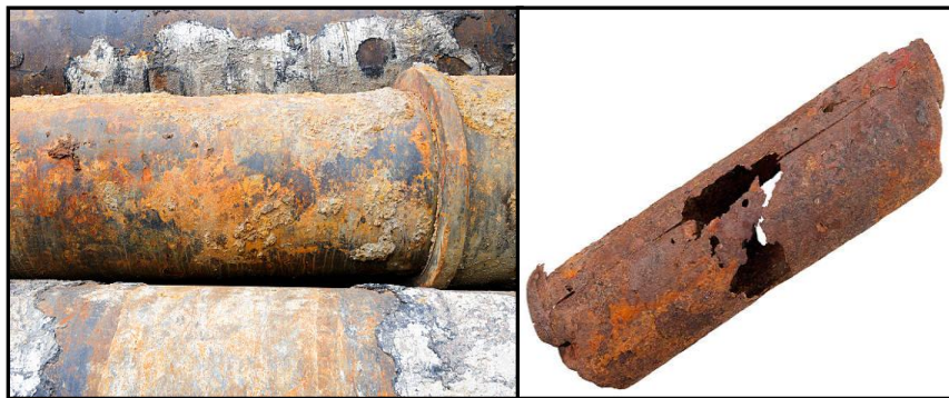
Figure 2.3 Steel Pipes affected by corrosion [187]
