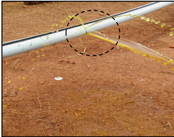
Figure 6.16 Pipe Spills due to damage
