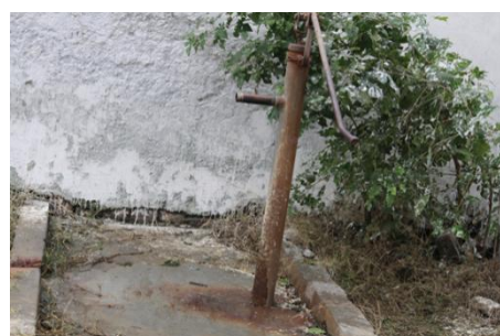
Fig. 4.38 Handpump in school and sanitation
