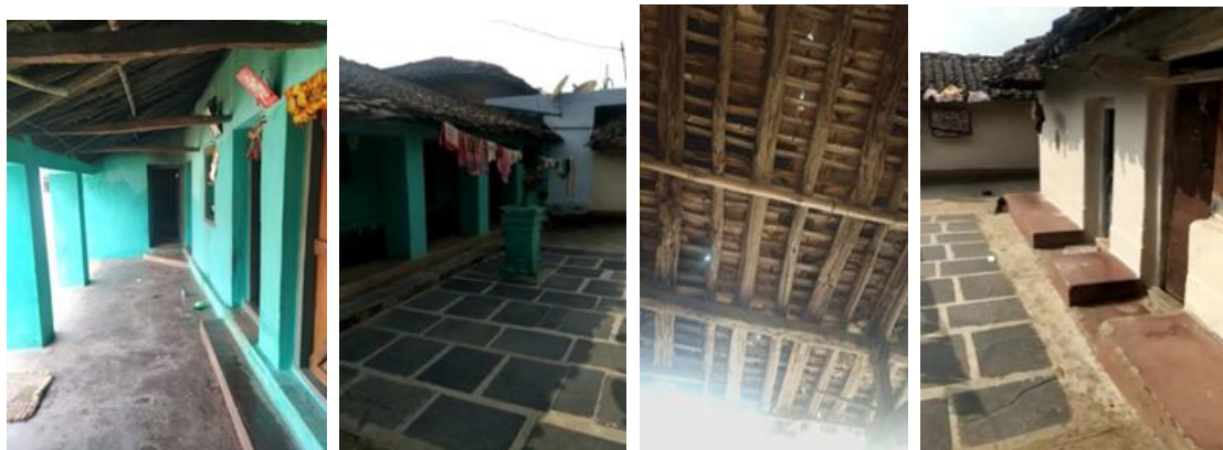
Fig. 256: Passage in Front of Dwelling Unit Fig. 257: Dwelling Unit on South Fig. 258: Timber Roof Fig. 259: Dwelling Unit on North
