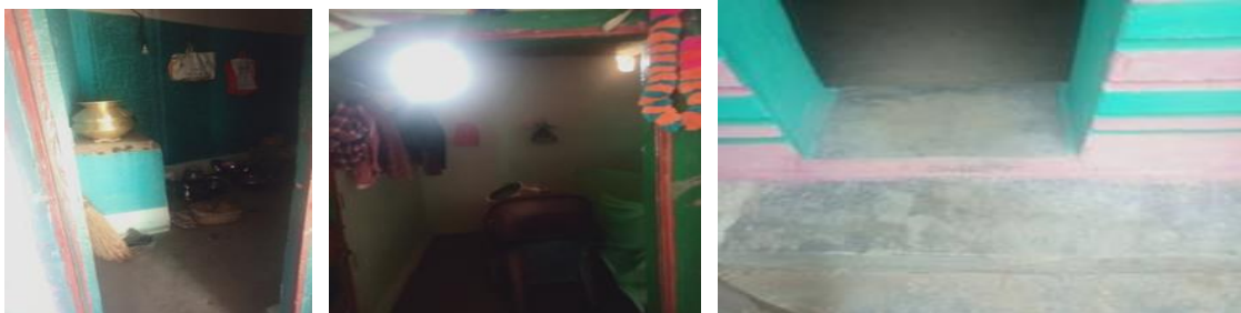
Fig. 161: Kitchen Fig. 162: Small Void for Ventilation Fig. 163: Cement Flooring with Level Difference
