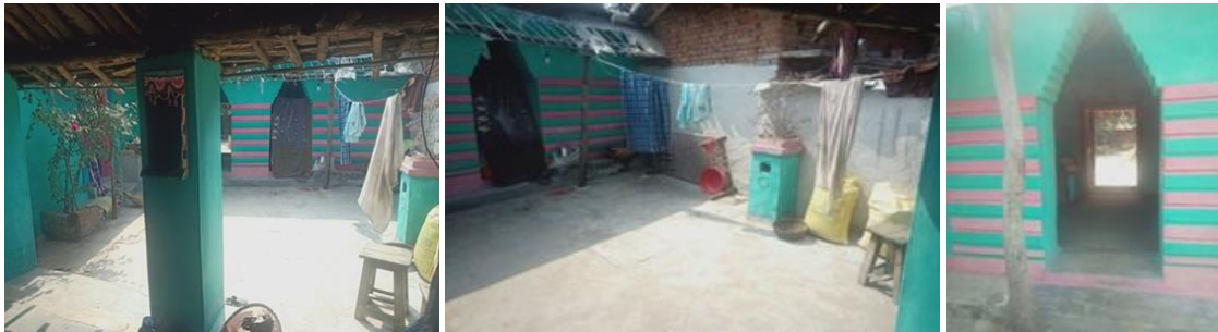
Fig. 158: View of Courtyard from Passage Fig. 159: Cement Flooring in Courtyard Fig. 160: Brick Corbelling
