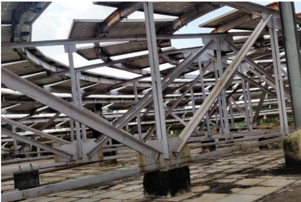
Fig. 123: Truss Support for Solar Panels
