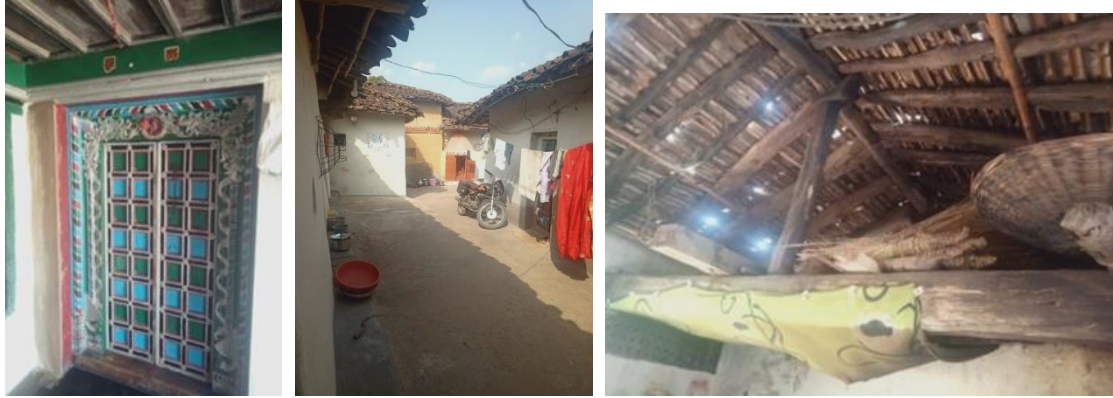
Fig. 239: Door of Kitchen Fig. 240: View of Rear Passage Fig. 241: King Post Timber Truss Roof
