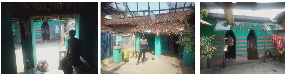
Fig. 164: Brick Pier Supporting Roof Fig. 165: Sloping Roof Fig. 166: Shade at Lintel Level
