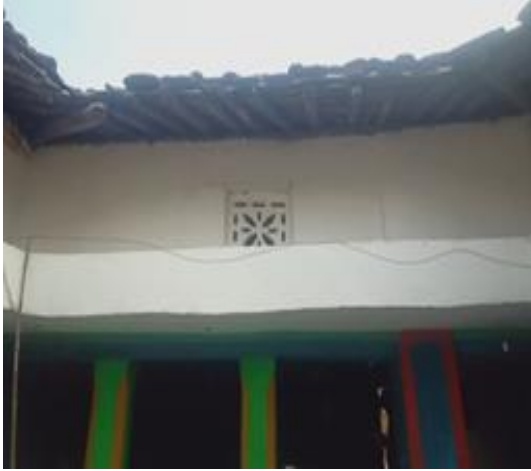
Fig. 190: Ventilator for Ventilation
