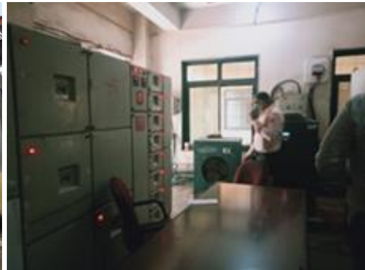
Fig. 124: Power Generation Room
