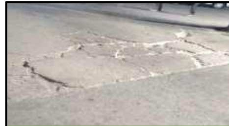
Fig.1.2 Failure of CC Pavement at Toll Plaza
