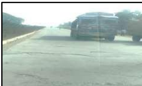
Fig.1.3 Failure of CC Pavement in a National Highway
