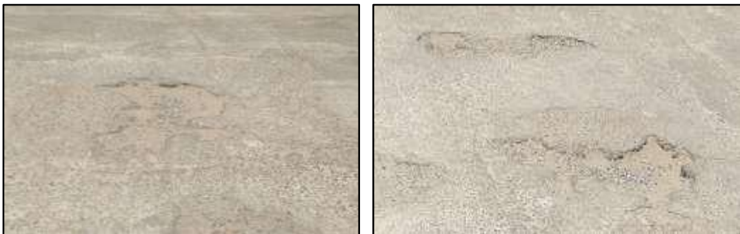
(a) CC Pot Hole depth 60mm to 80mm (b) CC Pot Hole depth 80mm to 100mm Fig.6.11 Pot Holes of various depths in CC Pavements
