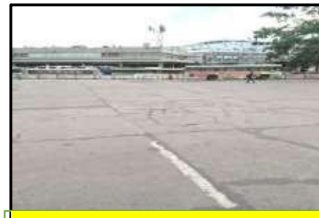
Fig.1.4 Failure of CC Pavement in urban area
