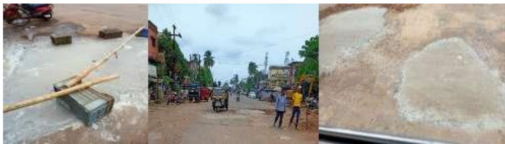
Fig. 6.15 View of CC Pavement potholes repaired with SCC HyFR-NA1.5 recipe at 356 days after repair- Patches were intact no damage observed
