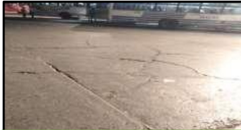
Fig.1.1 Cracking and Failure of CC Pavement at Bust Terminal
