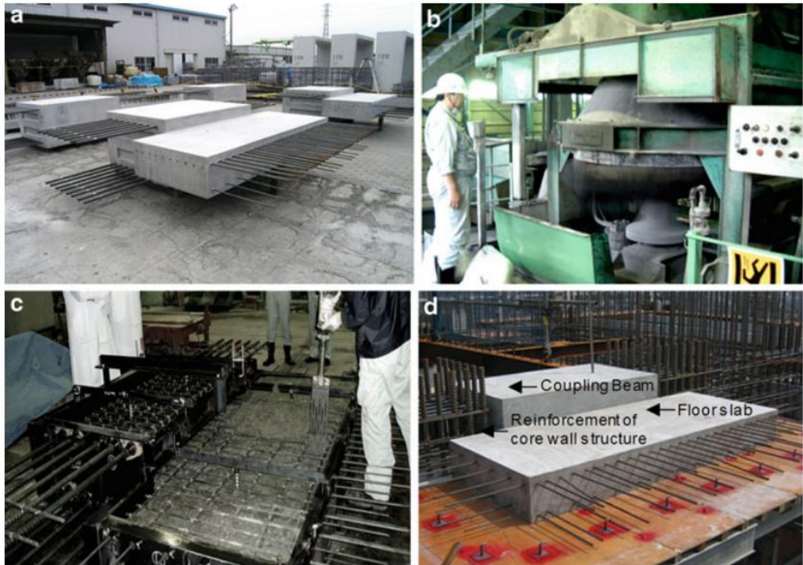
(a) ECC coupling beams, (b) Omni mixer mixing the fresh ECC, (c) Casting of ECC coupling beam together with partial floor slab, and (d) ECC coupling at the building construction
