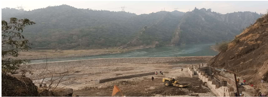
Source: Field work, 2023 Diverted flow of Ravi River downstream of Ranjit Sagar Dam due to ongoing construction of Shahpur Kandi Barrage
